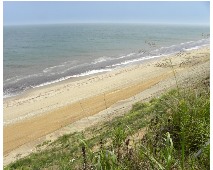
'Sconset beach with installed geotube system (Summer 2014).
