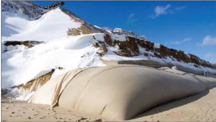
Exposed geotubes after the historic blizzard Wednesday protected the toe of Sconset Bluff.
