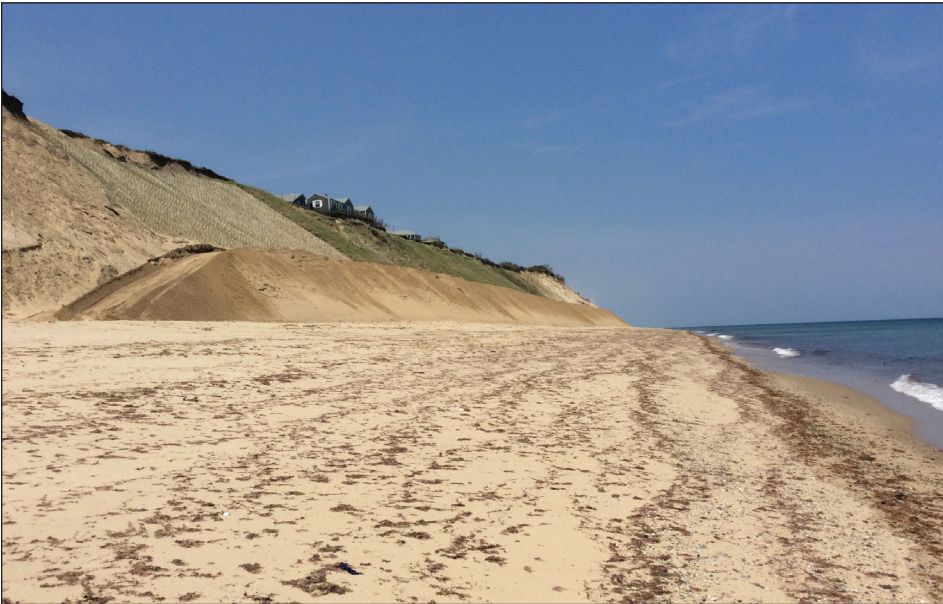
Sand-covered geotubes protect the toe of the bluff. Newly planted vegetation (foreground) and one-year-old vegetation (background) stabilize the face of the bluff. May 2016
