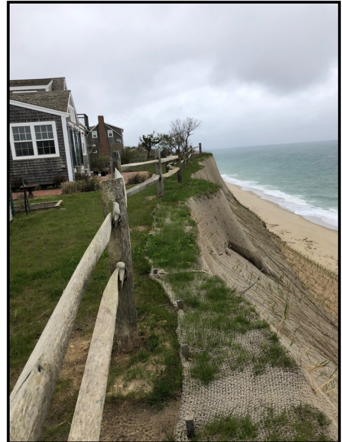
View of 109 Baxter Road facing north. Note the nearly vertical slope fronting this house.
