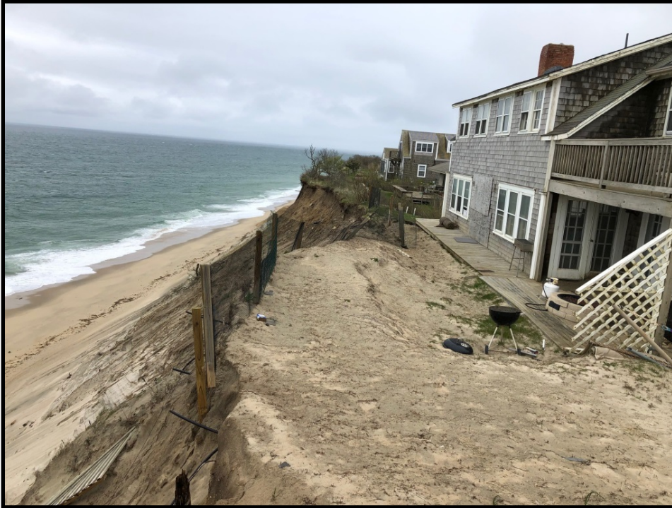
View of 115 Baxter Road facing south. Note steep un-vegetated slope fronting this house
